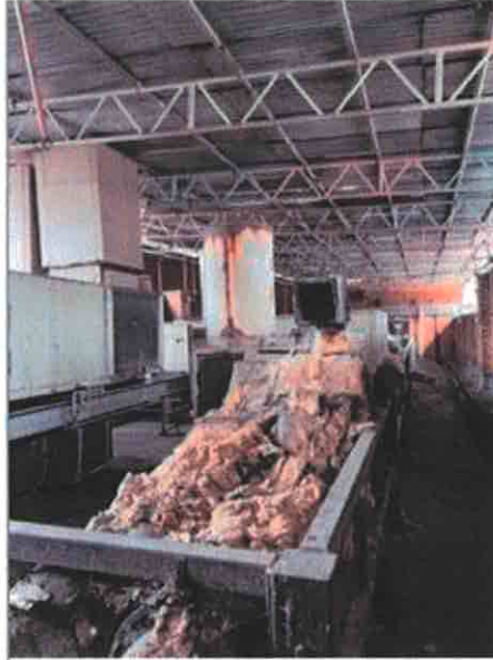
Plate No.1 View of the flat roof facing towards the rear of the building with A/C and other ventilation plant and electrical equipment
